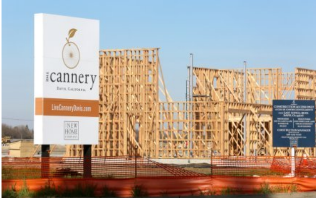
Walls for The Cannery's Barn are being framed at the site of the new development north of Covell Boulevard at J Street. Sue Cockrell/Enterprise photo
